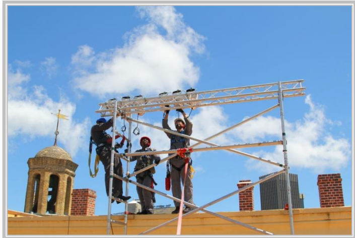
Photo 3: The crew from 3 Electrical Workshop have to re-install all the lights on the toppled tower
